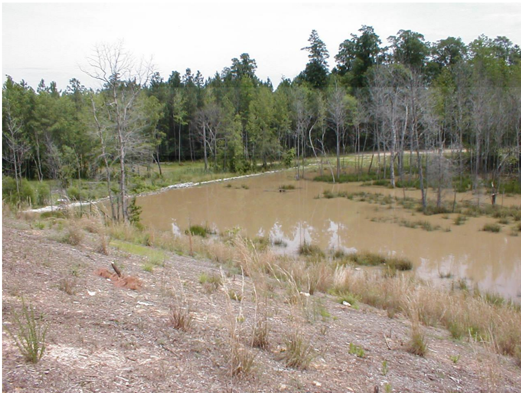
June 4, 2001 – Heavy sedimentation from the construction of Green Hope High School and Elementary School
